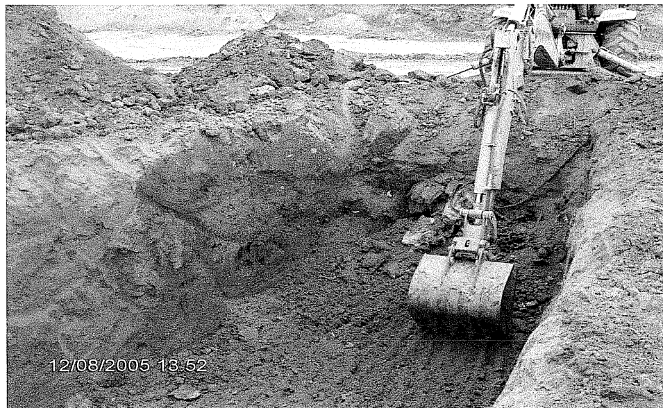
PHOTO 4 – Wellpad 1-10; trash fill excavation showing debris and hydrocarbon staining.
